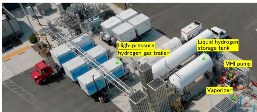
Figure 6 Hydrogen supply facility run by FirstElement Fuel
