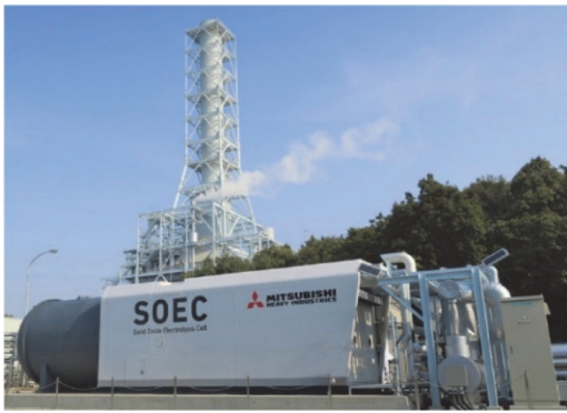
Figure 4 SOEC demonstration unit installed at Takasago Hydrogen Park
