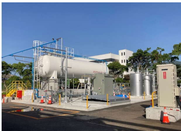
Figure 4 Appearance of ammonia supply equipment
