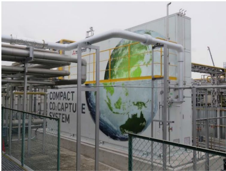
Figure 5 Small-scale CO 2 capture system (for gas engine)
