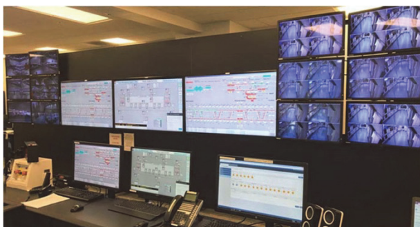
Figure 2 Central Control Room
