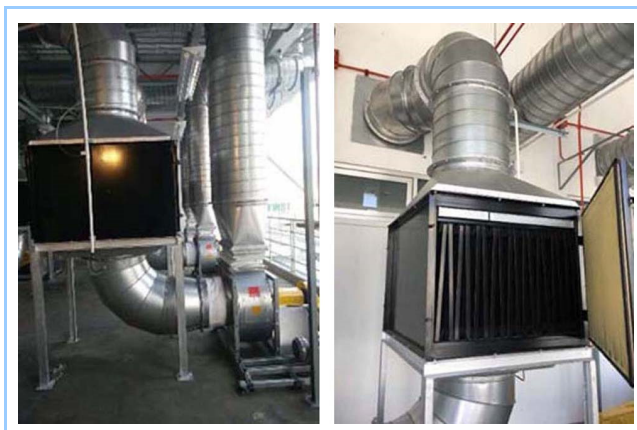
Figure 3 Activated carbon filters
