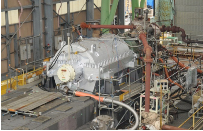
Figure 1 Performance test in propane refrigeration compressor
