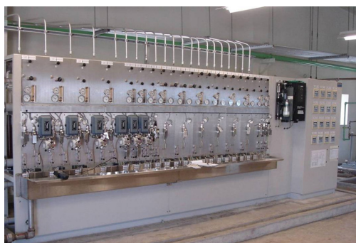
Figure 4 Sampling rack (taken at the No. 5 power plant)
