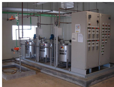
Figure 5 Dosing equipment (taken at the No. 5 power plant)
