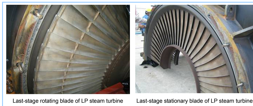
Figure 8 Low-pressure steam turbine during overhaul inspection (No. 2 power plant, August 2007)
