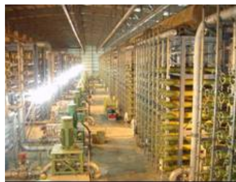
Figure 2 Low-pressure RO modules for the second and third passes
