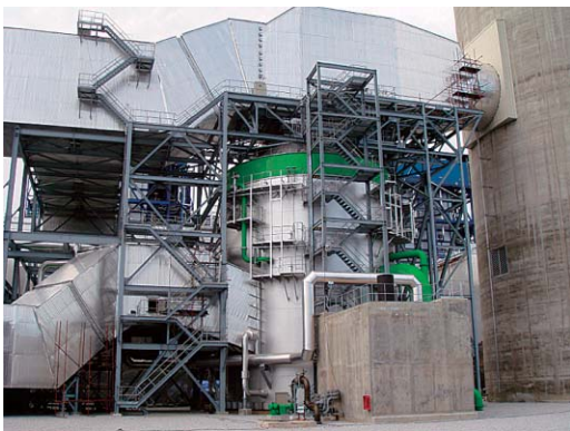
Fig. 7 Seawater desulfurization system (absorber)
