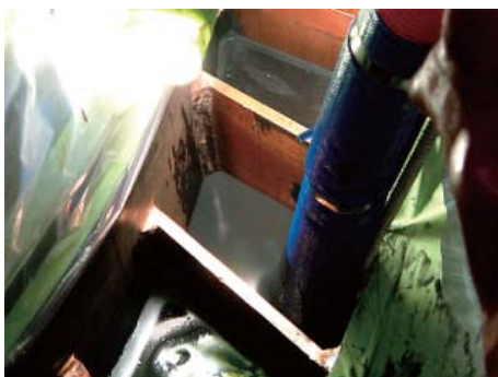
Fig. 6 Neutron shielding material, "MREX" Execution of the filling work between the main body shell of the cask and outer shell.
