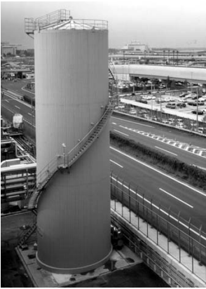
Fig. 14 PCM heat accumulator installed at New Tokyo International Airport
