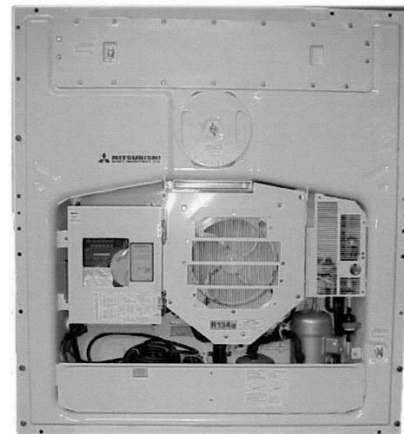
Fig. 13 External view of marine refrigeration unit
