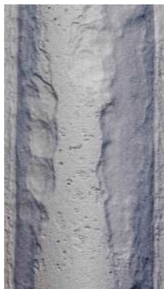
Figure 2 Example of damage to boiler heat transfer tube (sulfide corrosion, with outer surface scale removed)
