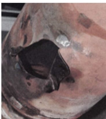
Figure 1 Example of damage to plant piping (flow accelerated corrosion (FAC))
