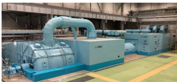
Figure 1 Appearance of turbine floor
