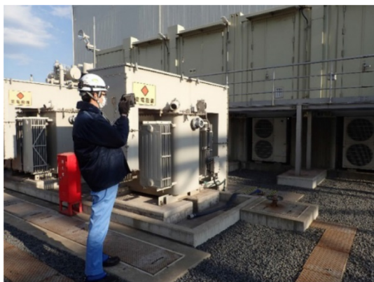
Figure 8 Trial of the smart patrol inspection system at a power generation plant
