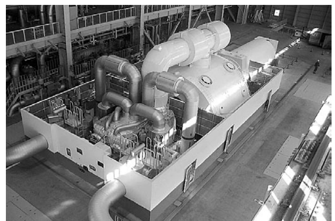
Fig. 2 External view of Hirono No. 5 steam turbine
