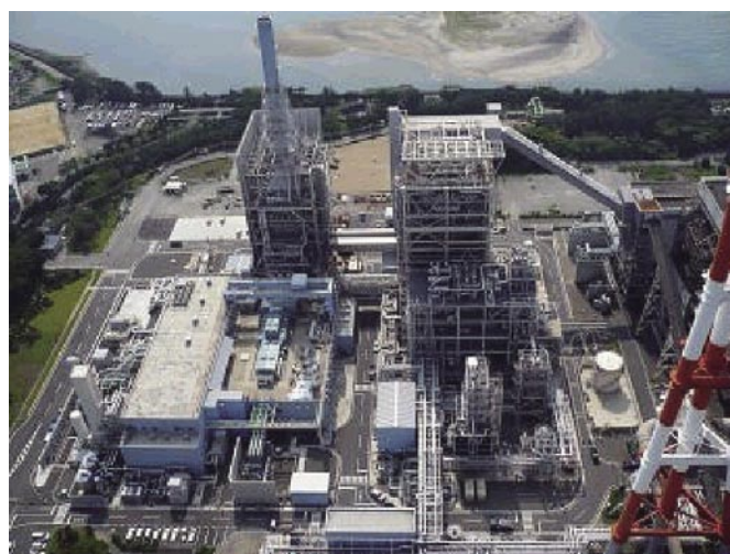
Fig. 6 250 MW class air-fired IGCC demonstration unit (Built by Clean Coal Power R&D Co., Ltd.)
