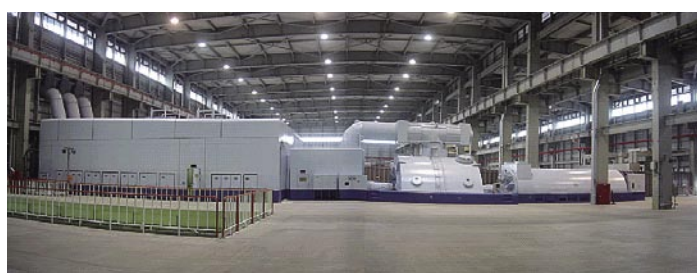
Fig. 7 1,500°C class GTCC plant (Kawasaki Thermal Power Station No. 1 Series of Tokyo Electric Power Company)
