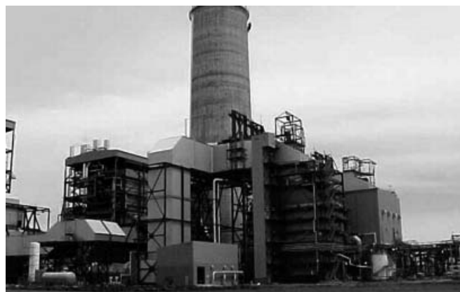
Fig. 8 Absorber and auxiliary equipment of Ratchaburi Thermal Power Plant No.1 unit
