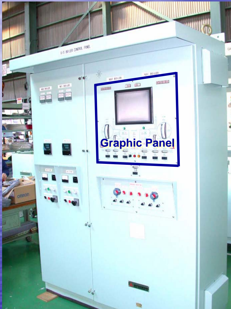
Local Boiler Control Panel
