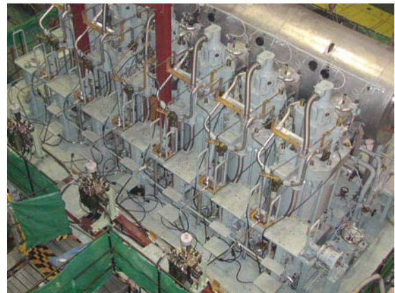
Figure 22. Water injection system installed in 6UEC50LSE
